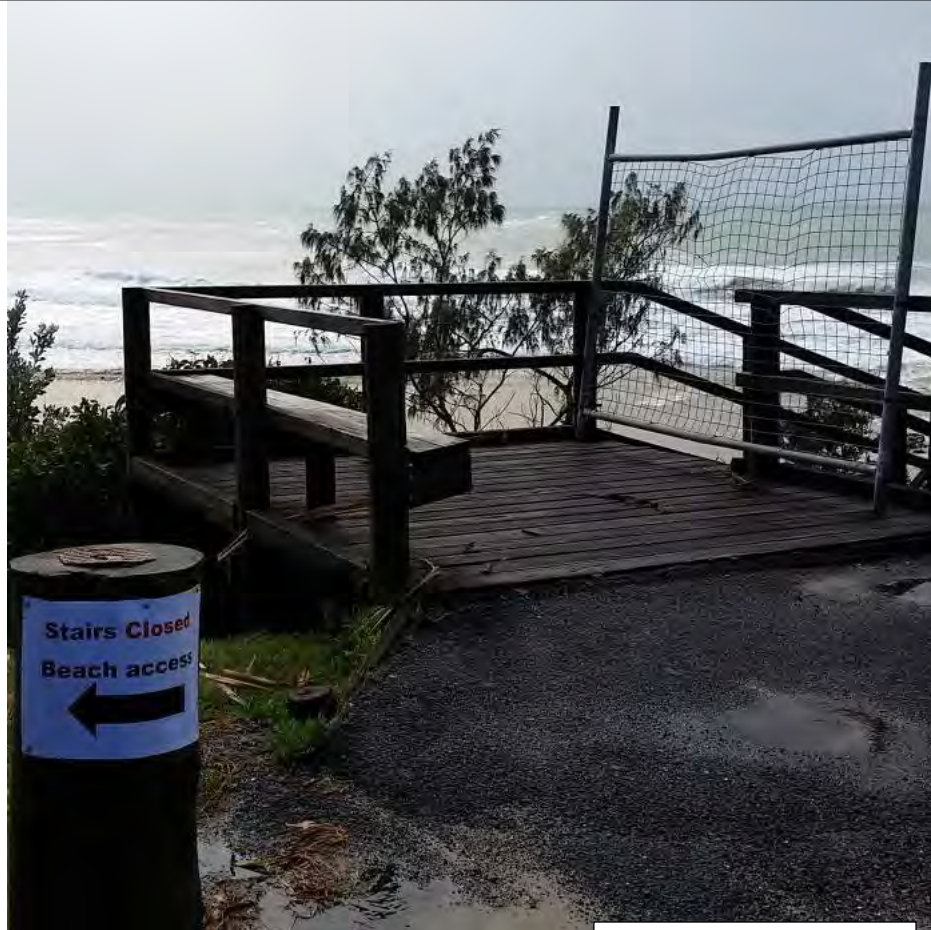
Storm damage Ocean View Headland
