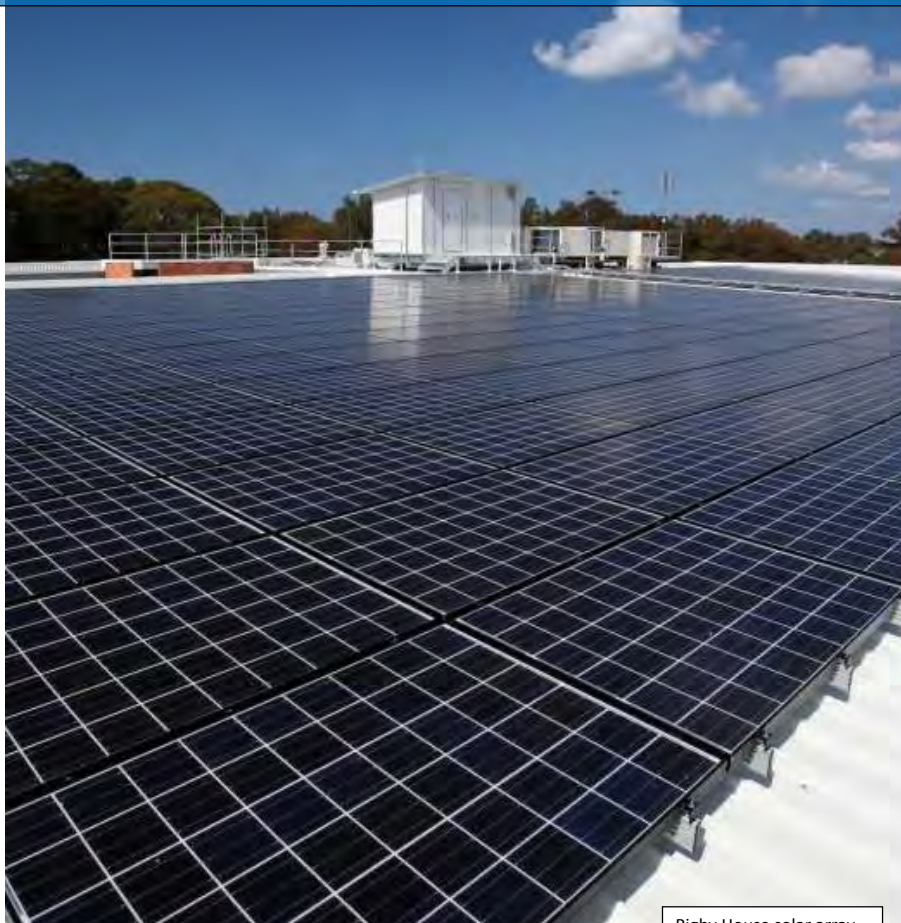
Rigby House solar array
