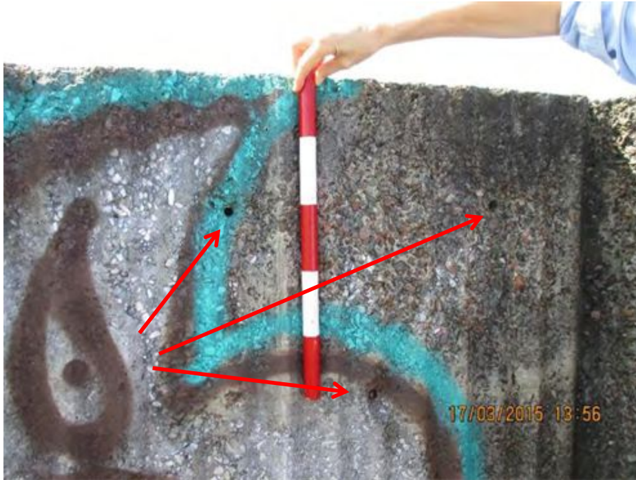
Plate 14. Northern wall of the rear compartment, showing three small holes in the concrete.
