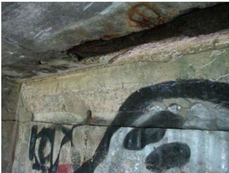
Plate 8. Large fragments of concrete missing from the roof of the structure, exposing its metal lining.
