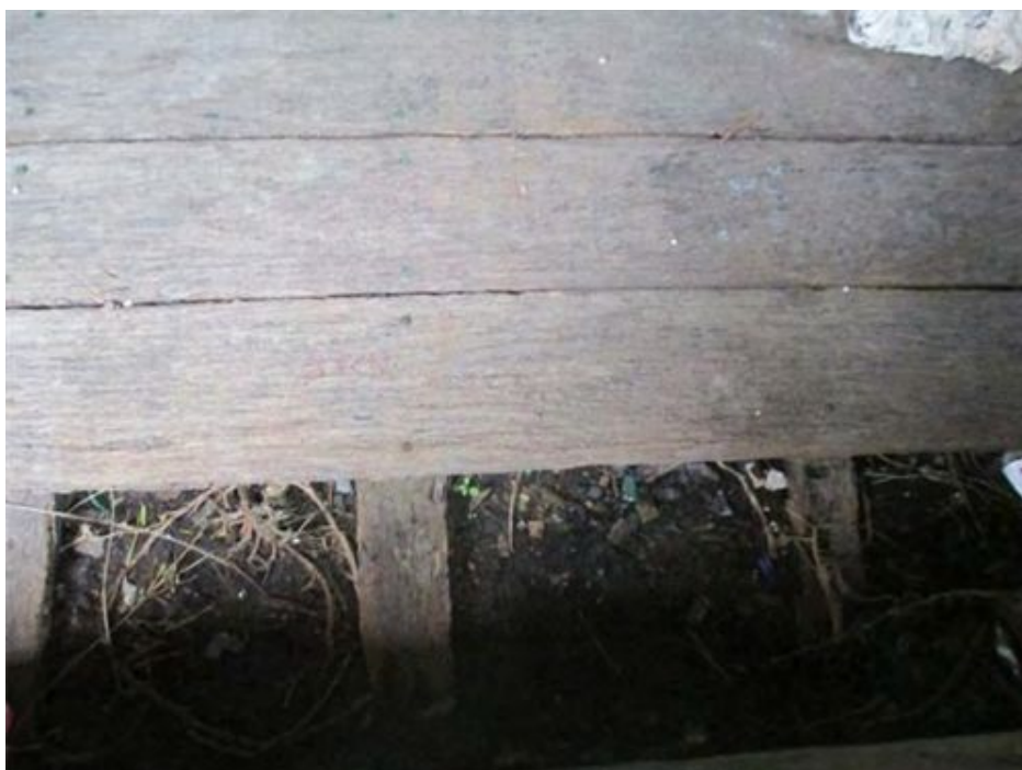
Plate 9. Floorboards missing within the front compartment of the item.
