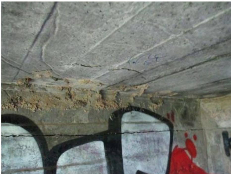
Plate 7. Large cracks noted in the walls and roof of the structure.
