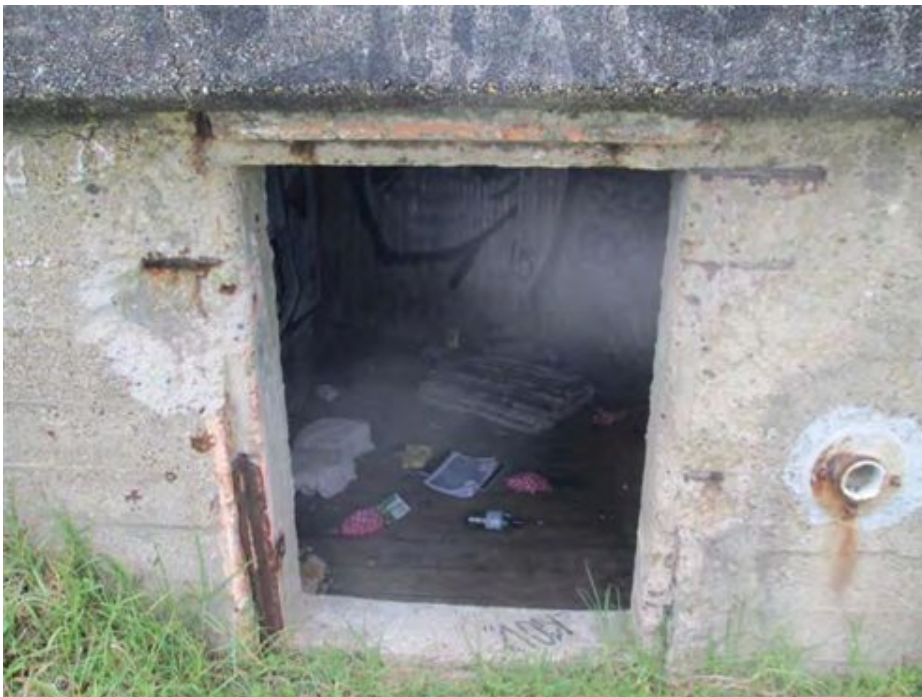
Plate 5. Remnants of metal hinge of former door + circular opening that connects to a similar opening on the inside roof.
