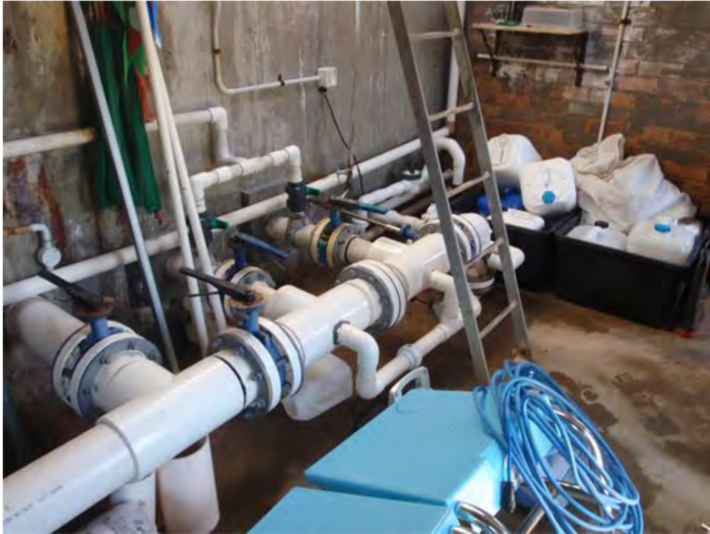
Picture 2 Showing current plant pipework
