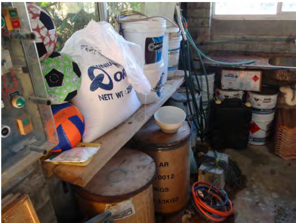
Picture 3 Showing current chemical storage within plant room
