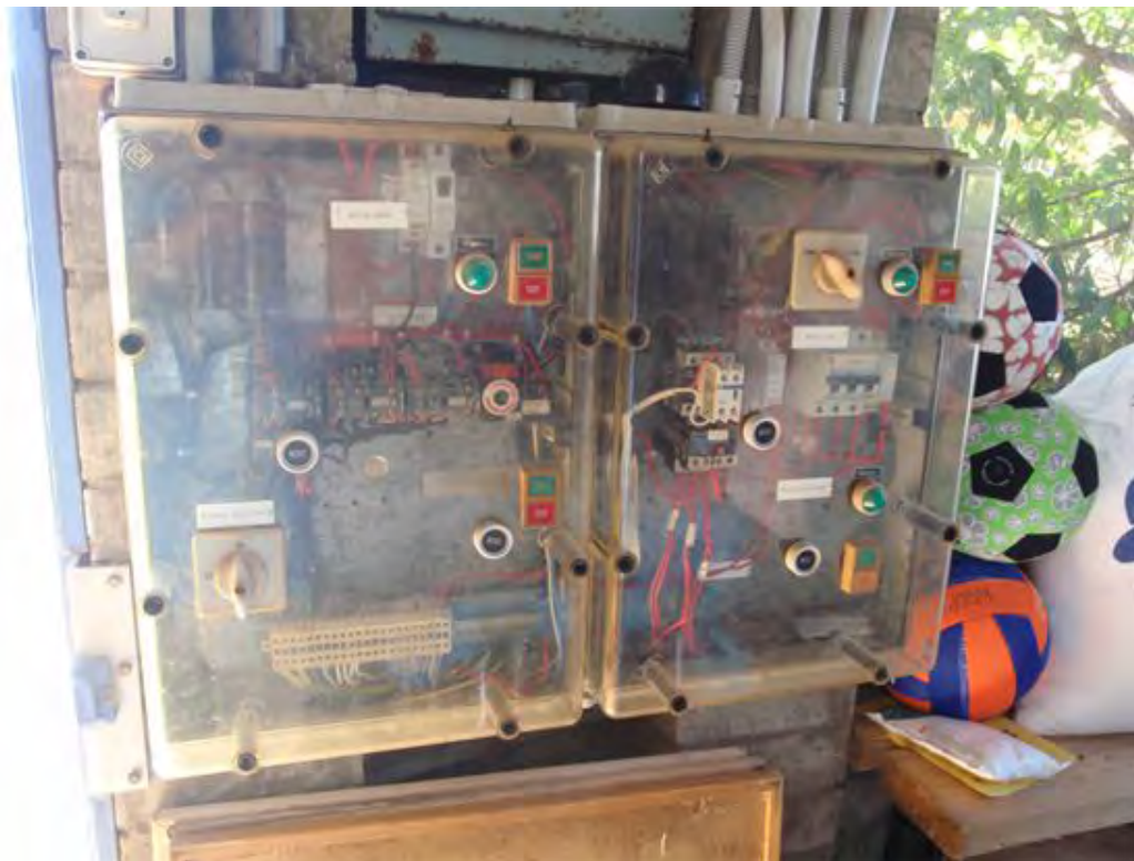
Picture 5 Showing current electrical control panel within plant room
