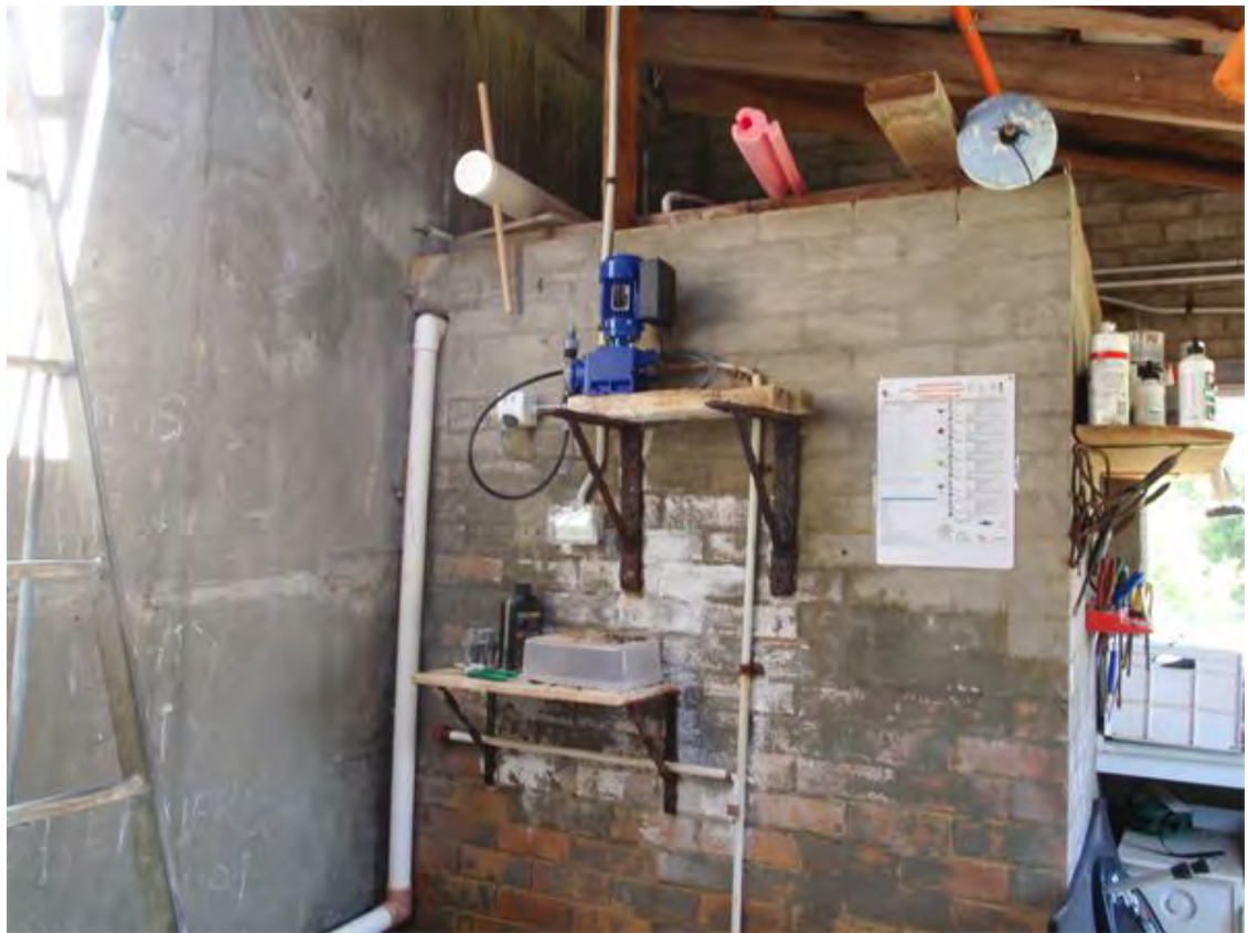
Picture 4 Showing liquid chlorine pump and container brick bunding around the storage tank.
