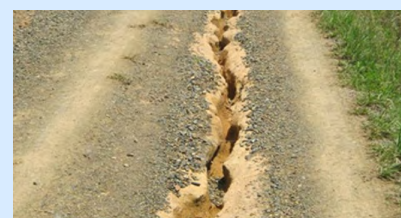
A flood-damaged road in rural NSW.
