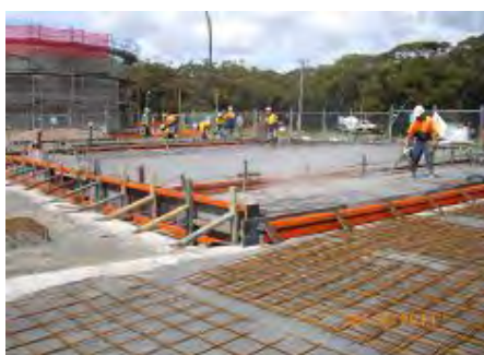
Constructing a multi-million dollar recycled water plant to reduce demand on community water supply. The project is partially funded by Federal grants.
