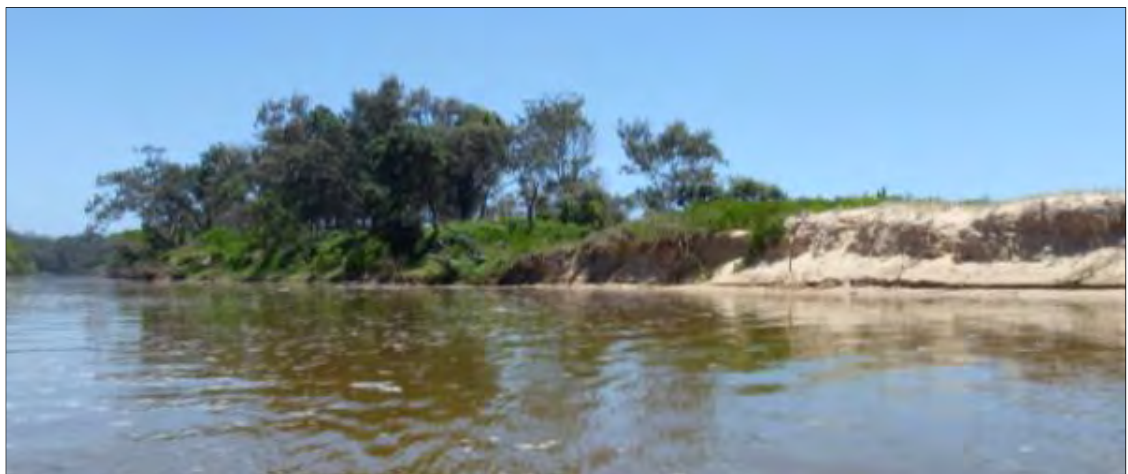
Plate C.3 Bank Erosion - scour and undercutting, lower Darkum Creek – left bank (looking north)
