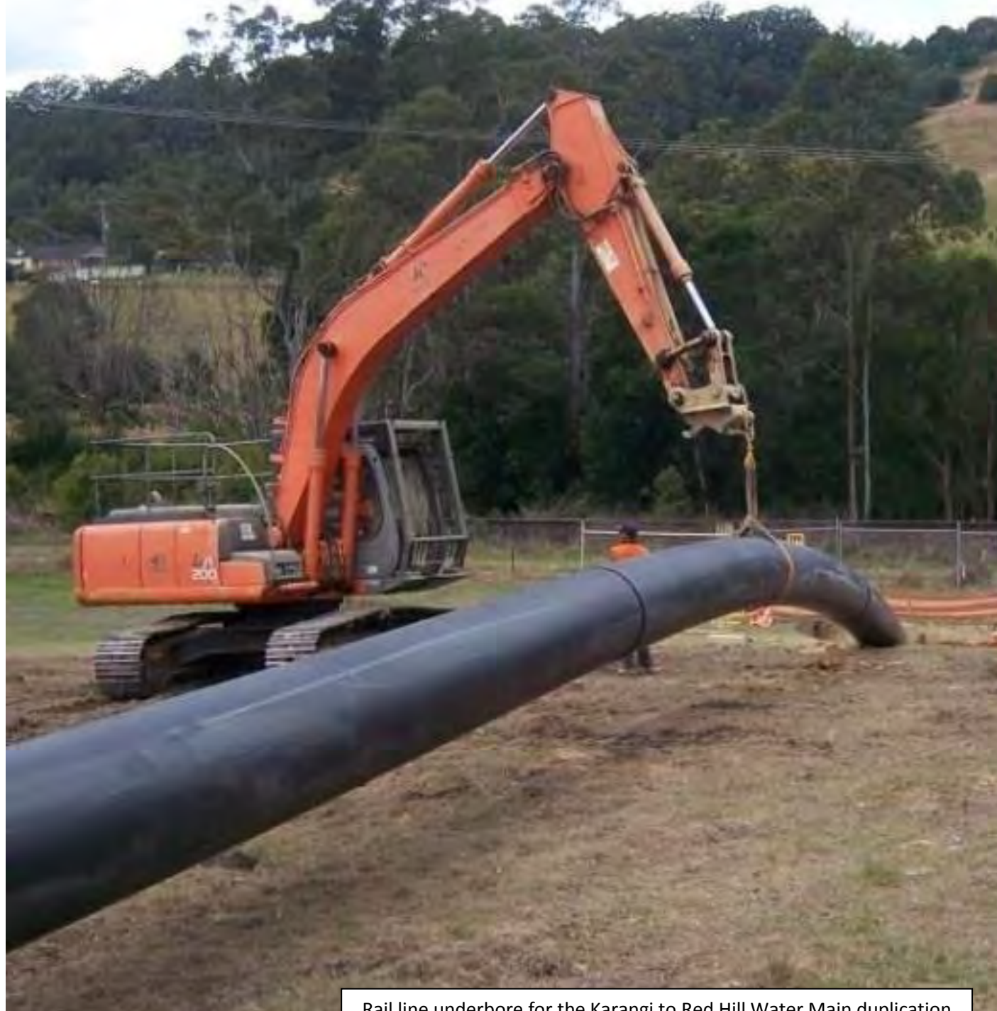
Rail line underbore for the Karangi to Red Hill Water Main duplication
