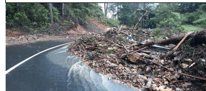
Eastern Dorrigo Way debris removed – February 2020
