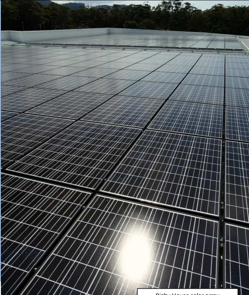
Rigby House solar array
