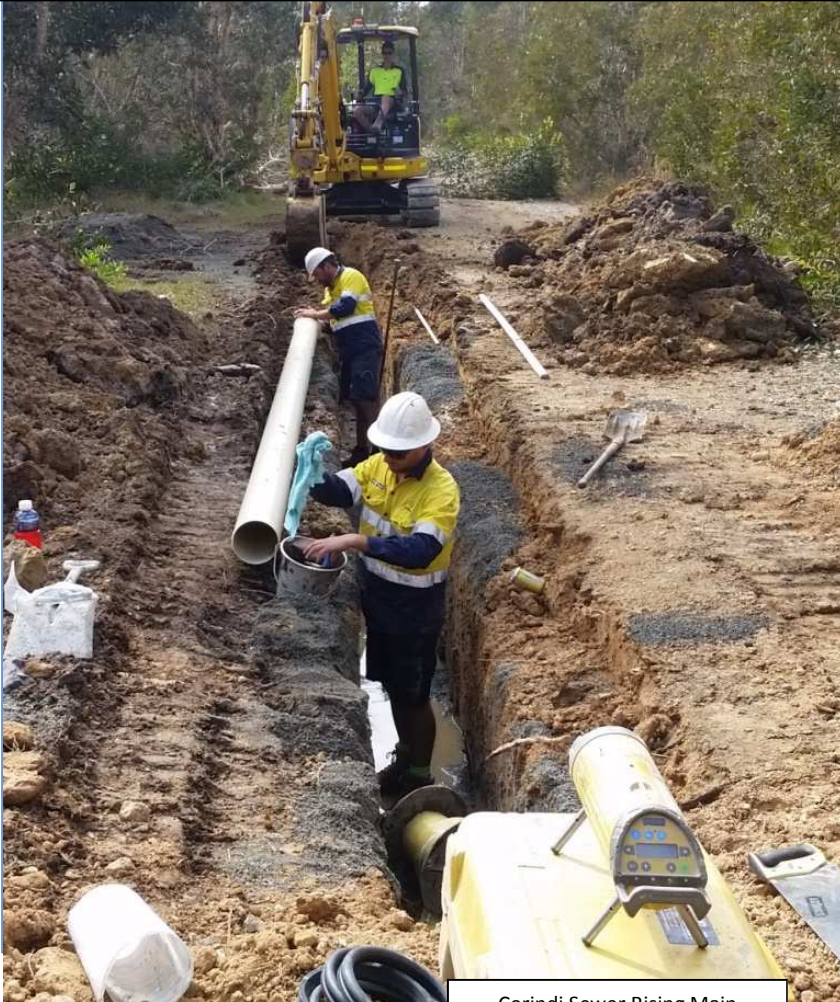
Corindi Sewer Rising Main
