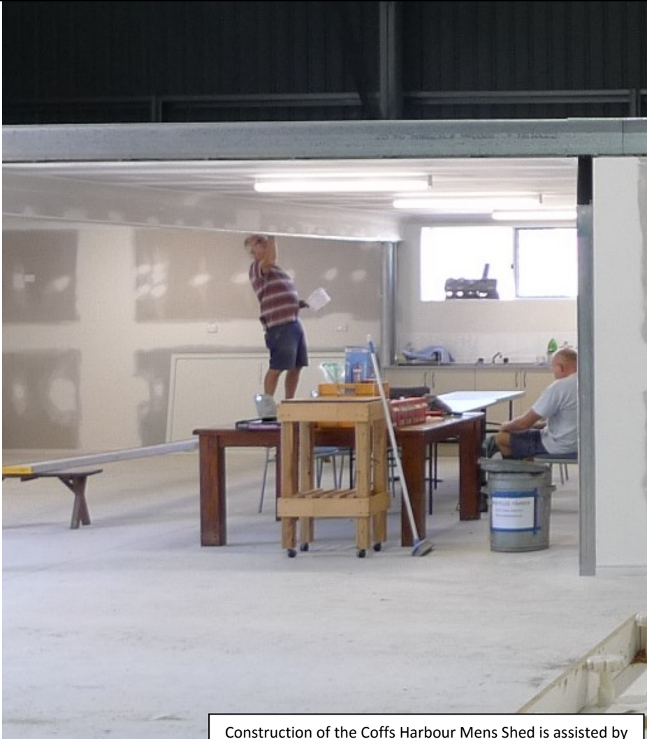
Construction of the Coffs Harbour Mens Shed is assisted by Councils' Community Capital Infrastructure Grants program
