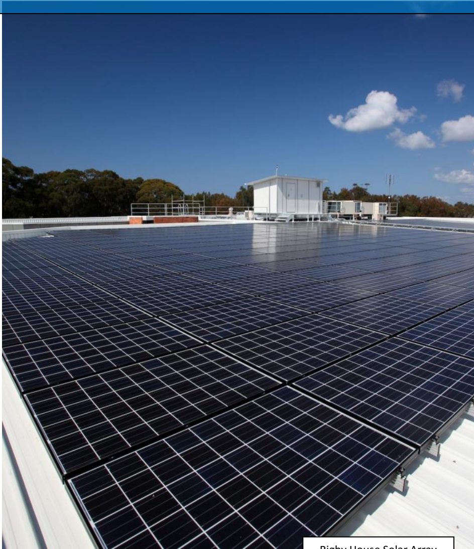
Rigby House Solar Array
