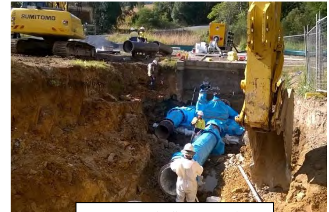
Karangi-Red Hill Water Pipeline
