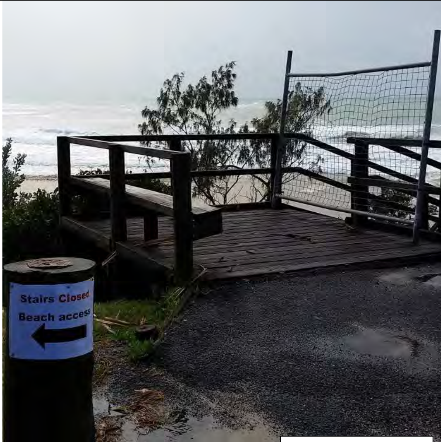
Storm damage Ocean View Headland
