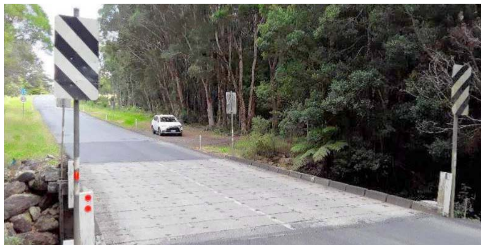
A 40kph speed limit is currently applied to Little Nymboida Bridge due to safety concerns.
